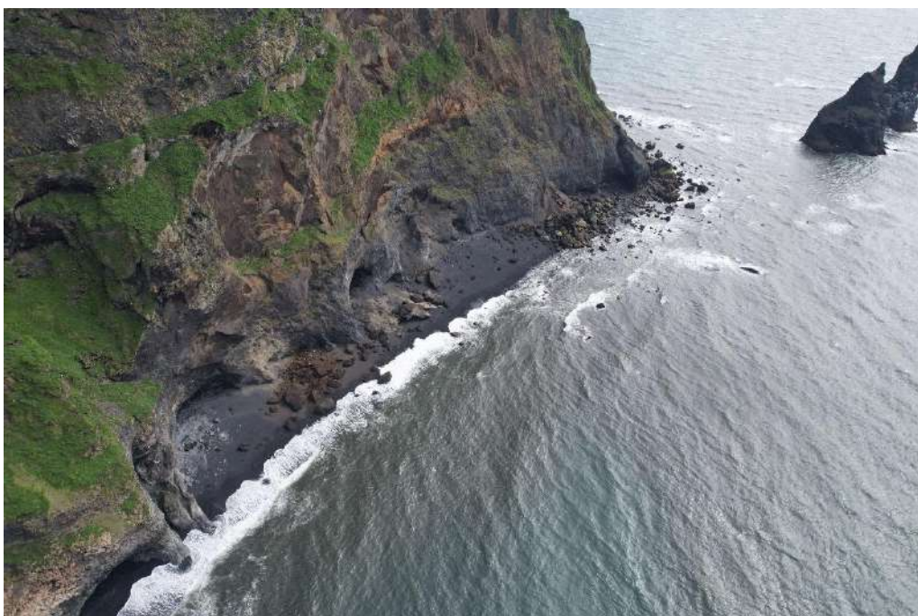
Figure 11 shows the cliff face of Reynisfjall at 11:11 on the 15 th of June. Fresh debris can be seen on the rocks on the left and the scar on the cliff can be seen as well.
